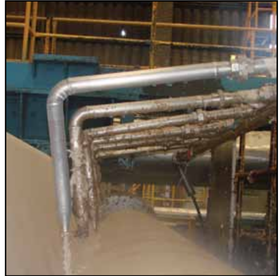
(Above): The foremost pipe is covered in a .020" thick FEP sleeve. Note the difference in build up between the FEP covered pipe and the uncoated pipes.
